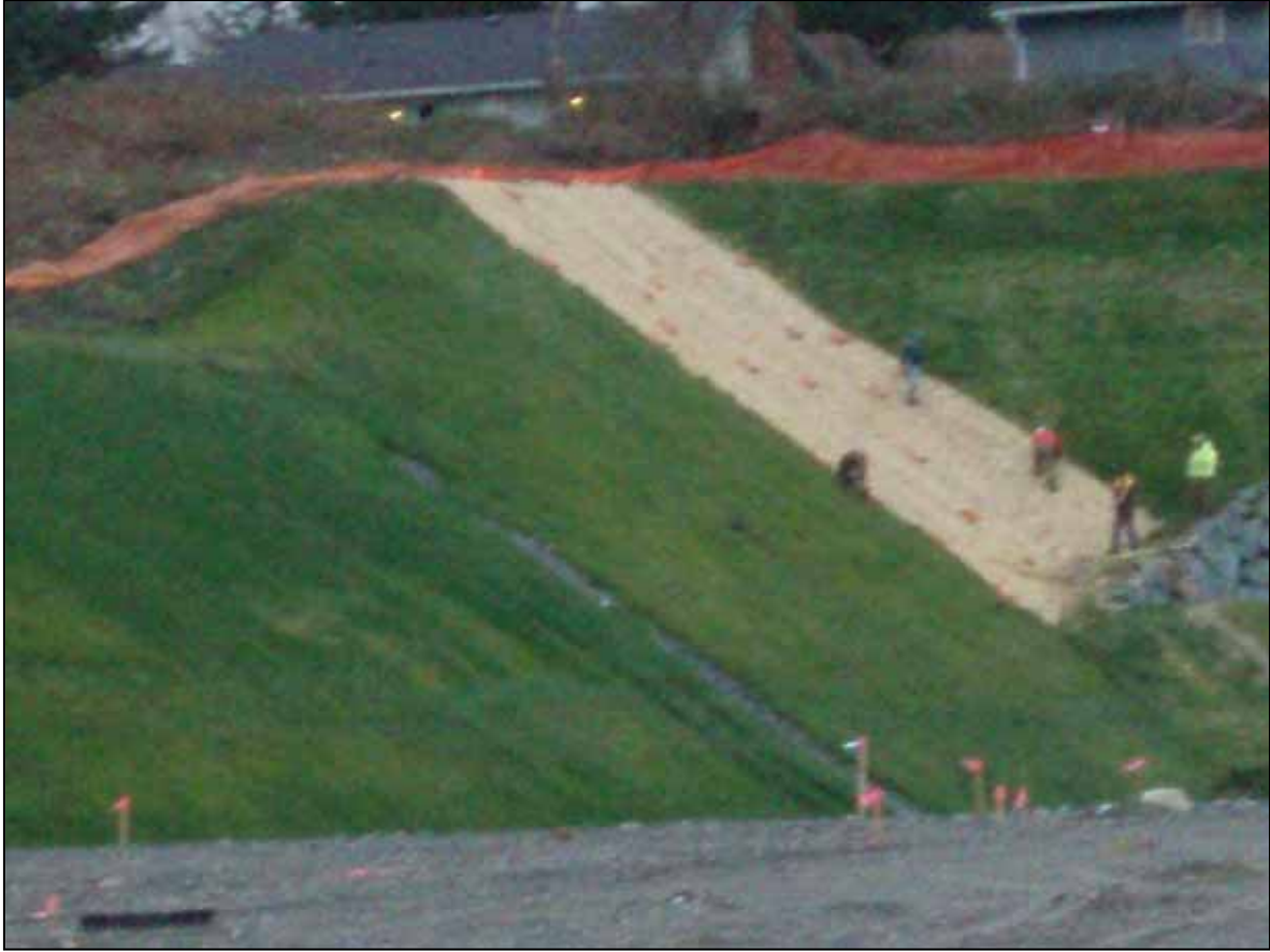
Photo 5. Reach 14. Crew works at northeast corner of development. Black tarp has been removed. Steward and Associates staff observed continuous groundwater flow emerging from the area one week prior to the date this picture was taken.
