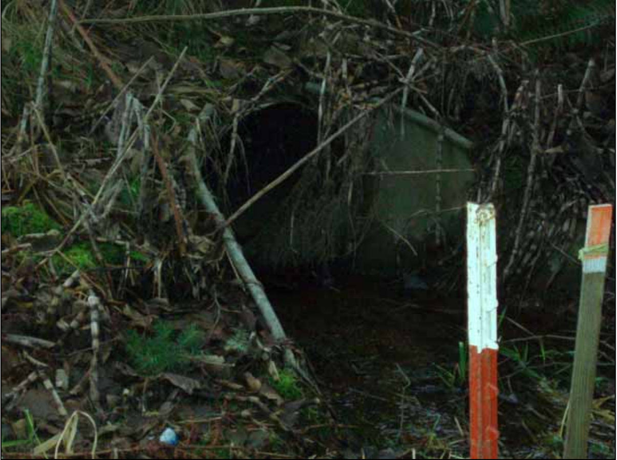
Photo 3. Reach 16. Myrick Fork, along with stormwater from SR9 and US2, enters 24 inch corrugated metal culvert leading under eastbound US2 off-ramp to stormwater pond.
