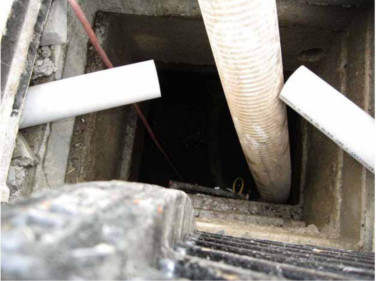
Photo 7. Reach 14. Eight inch plastic pipe pumping Snohomish Station project stormwater from the west to east end of the project site to infiltrate as groundwater.
