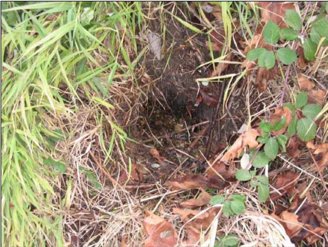
Photo 17. Reach 5. Myricks Fork emerging from embankment on east side of Bickford Avenue.
