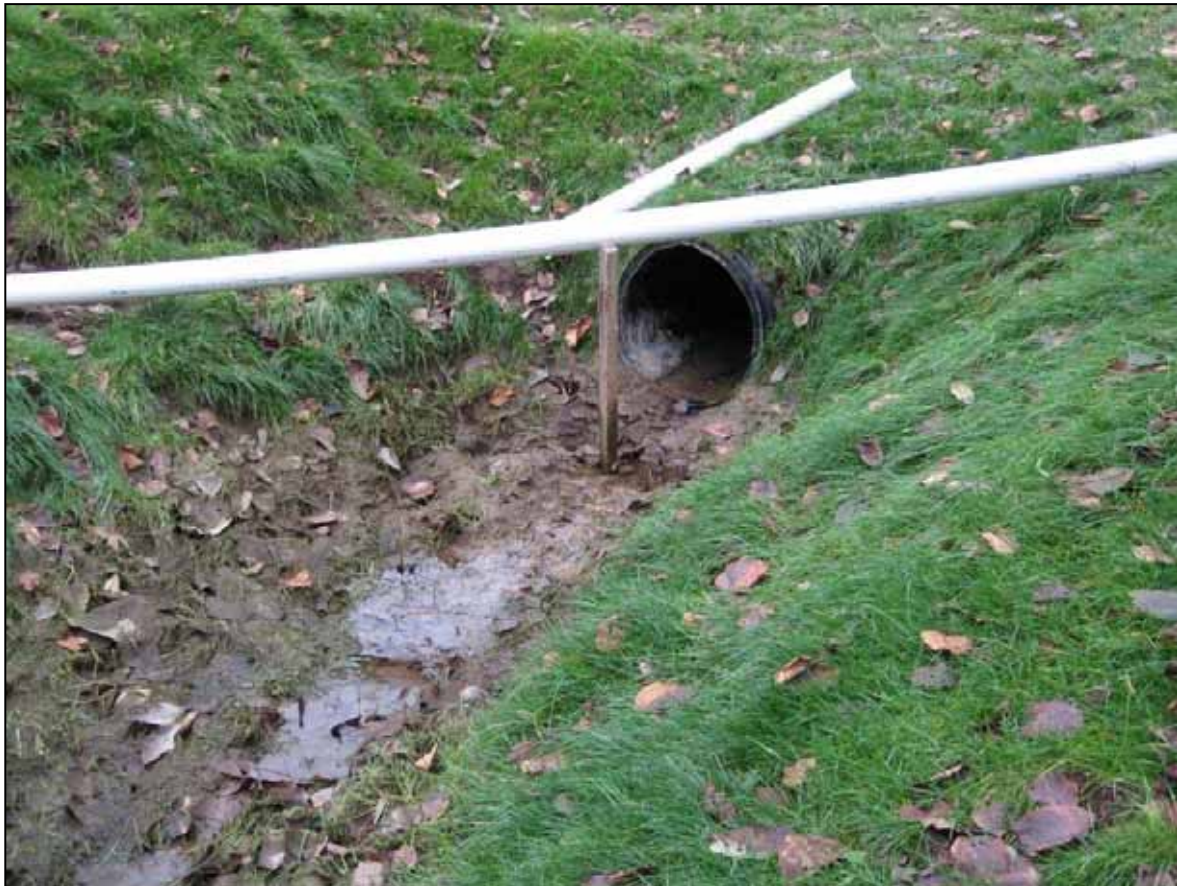
Photo 8. Reach 13. Black plastic pipe, 25 inches in diameter, at the southeast corner of Snohomish Station project.
